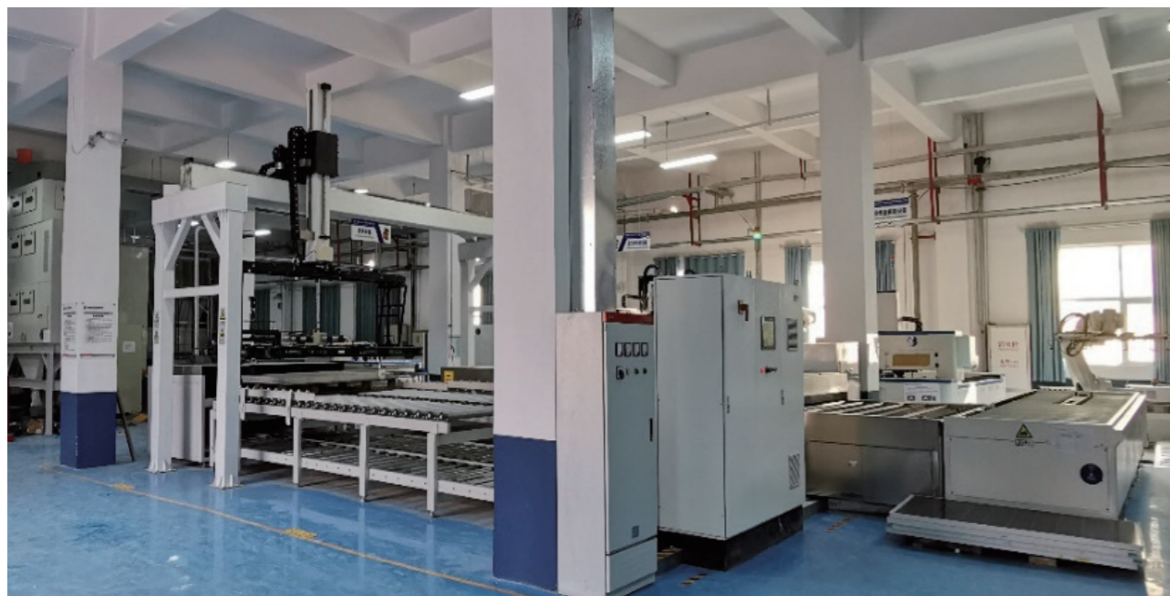
Figure 8-10 Demonstration Project for Recycling Decommissioned Crystalline Silicon Photovoltaic Modules (30 MW/year)
